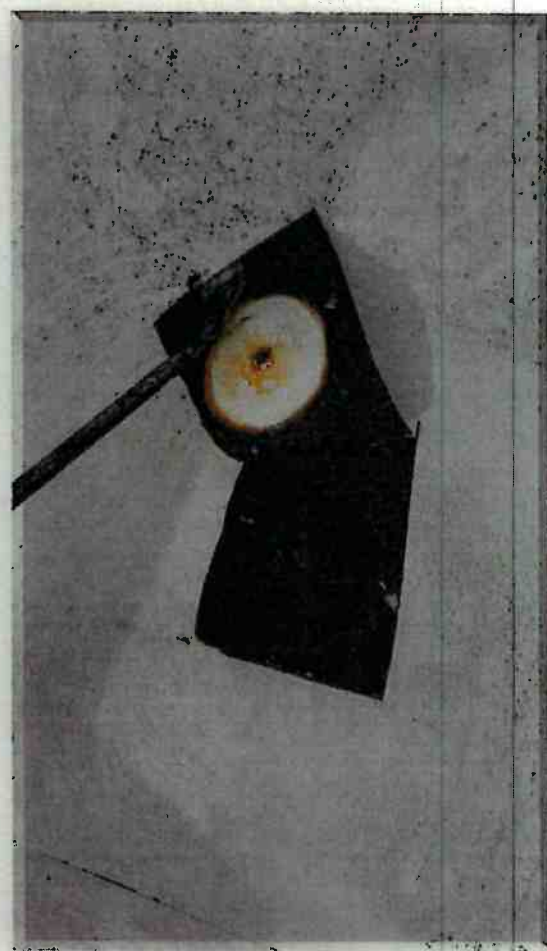
Photo 76 - Membrane glued to paper backing. Plate & screw fastening insulation to the concrete deck.
